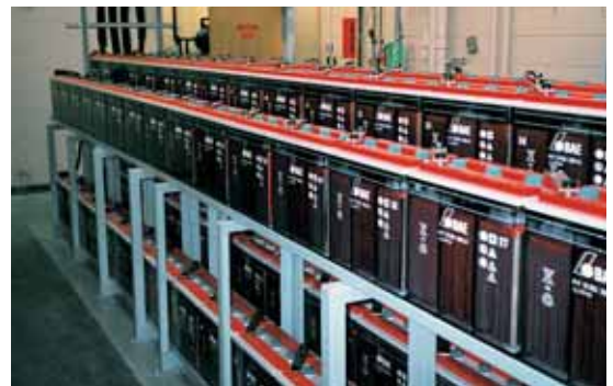
UPS application in USA 6 V 11 OGi 275
